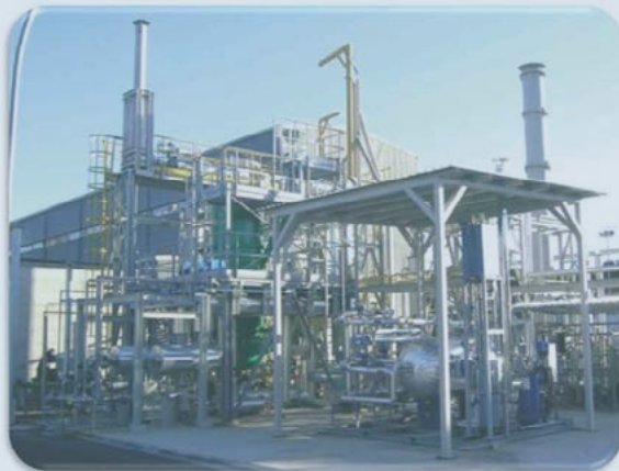
ZECOMIX is an European research infrastructure focused on hydrogen production from conventional fuels, present in Research Centre Casaccia of ENEA. This plant provided the benchmark values for the thesis.
